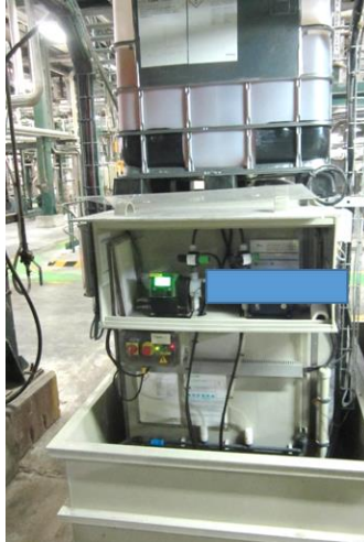
Figure 5: IBC with liquid enzyme on their secondary containment; example of mother-daughter decanting system
